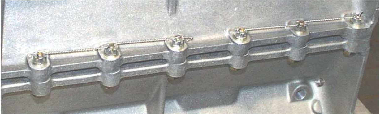
Figure 91 Safety Wire on the Nuts in the Crankcase Oil Sump
